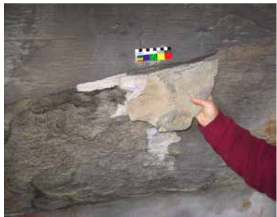
Figure 8. WW03 Recently exfoliated piece located on floor of shelter.
