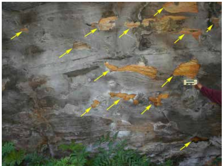
Figure 4. Detail of fire damage to the rear wall of BR21. Image courtesy of Melanie Thompson, BIOSIS Pty Ltd.
