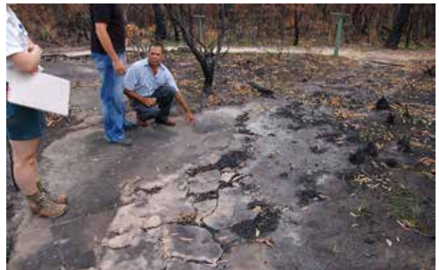
Figure 3. The same site after the fire. Note that damage to the sandstone is confined to the location of the former boardwalk.
