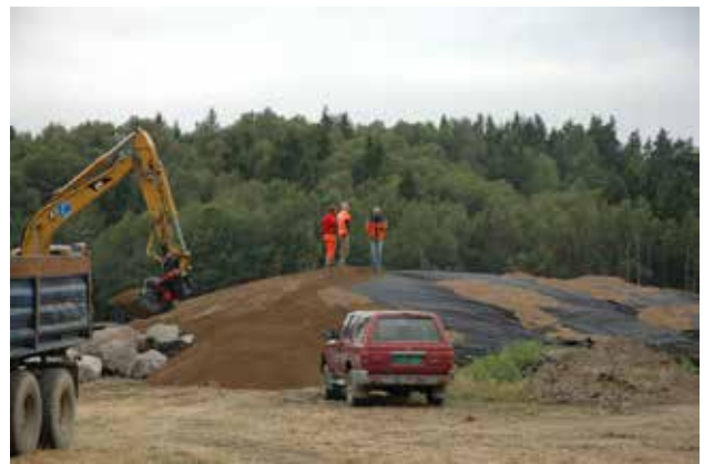
Figure 9. The geotextile (black fibre cloth) covers the layer of marine clay, and the dumping of natural gravel is under progress. Photograph: Gro Anita Bårdseth.
