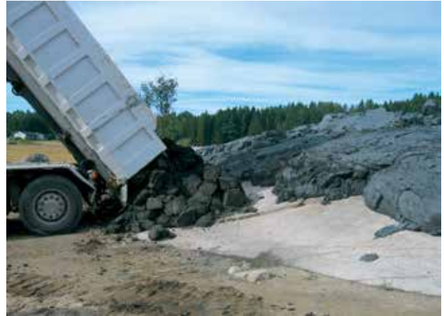
Figure 8. Dumping of dry clay in front of the marine clay, for the construction of supportive fillings. Photograph: Kristin Marie Berg.
