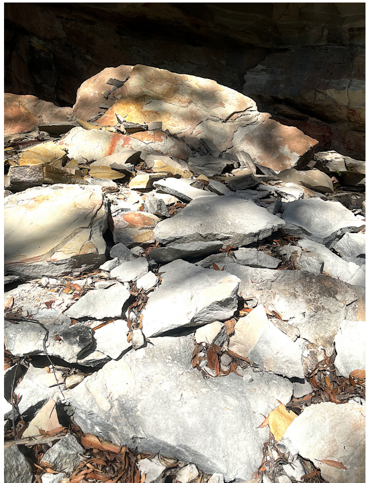
Figure 3. Thermal fracturing at Baloon Cave led to more painted rock surface sheeting off to the ground. Image: MK March 2022.
