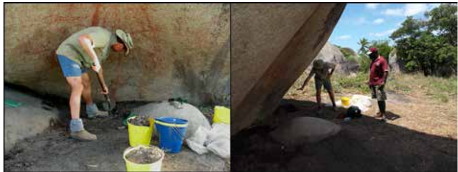
Figure 15. Left: preparing the ground surface for application of termiticide; right: discussing the application procedure with Dauan AQIS officer, Kevin Akiba.
