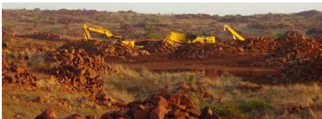
Destruction of Dampier rock art site at Holden Point on 7 February 2007; photograph taken secretly.
